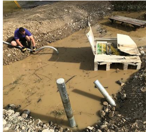
FDH 4021, damaged during flooding
